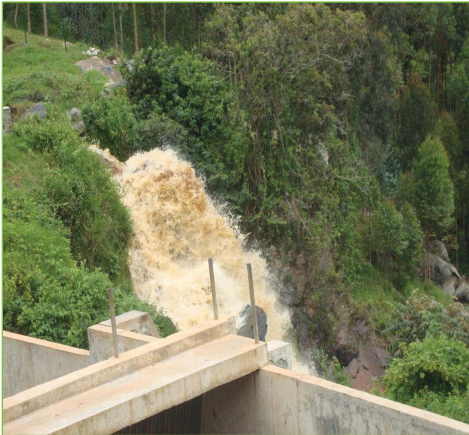
Micro hydro power unit in Butaro Sector, Burera District
