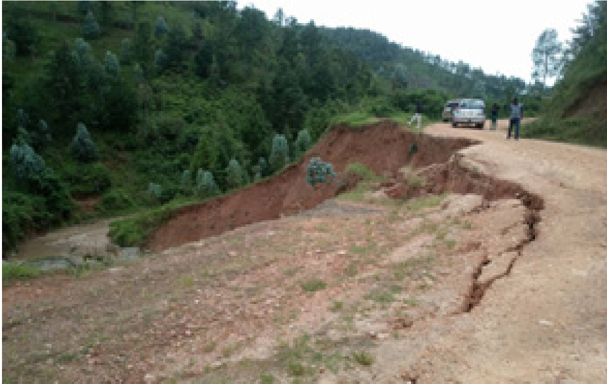
In the photo: a road which is continuously damaged by floods and rendered impassable
