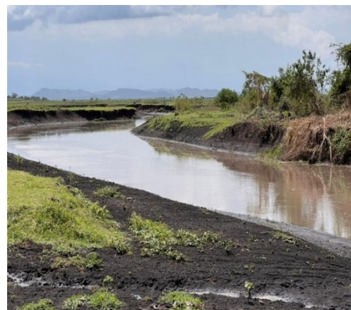
Figure 19: Nyamonyo River constantly floods and makes access to Wegero village difficult
